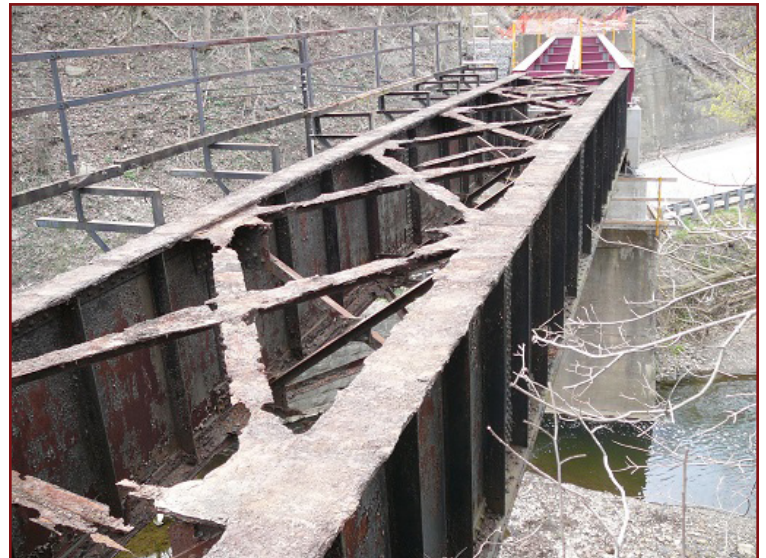
This view of a bigger bridge with deck removed shows the similar construction with main plate girders and cross bracing on a much larger scale. Note the brackets and railing for a safety walkway on the left side of the span.
