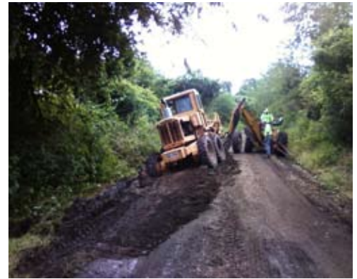
Bill Capp checks over Frank Ludwin's grading and digging. (Photo- John Kozak)
