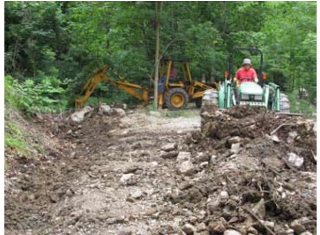
Bill Capp, a trail volunteer, using the trail tractor to move fill material.
